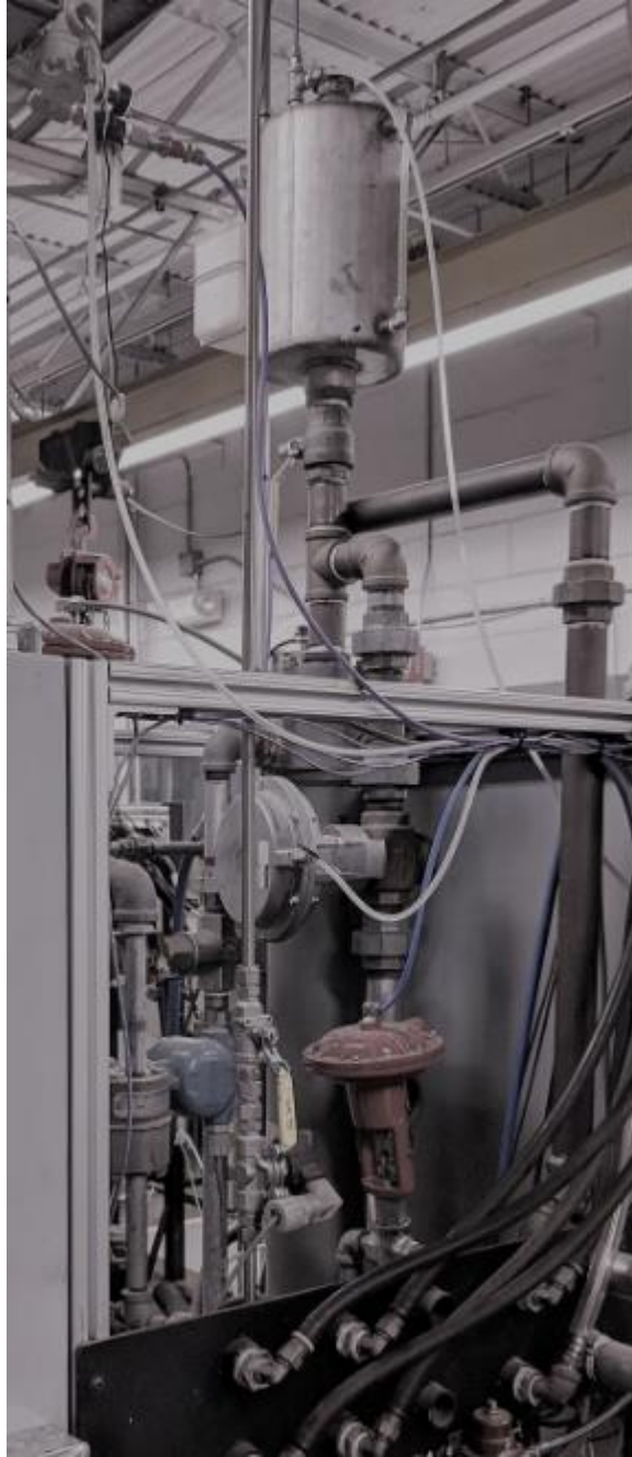
FIG. A7.23 Typical Cooling System, Flow Control Valve, Reservoir and Sight Glass
