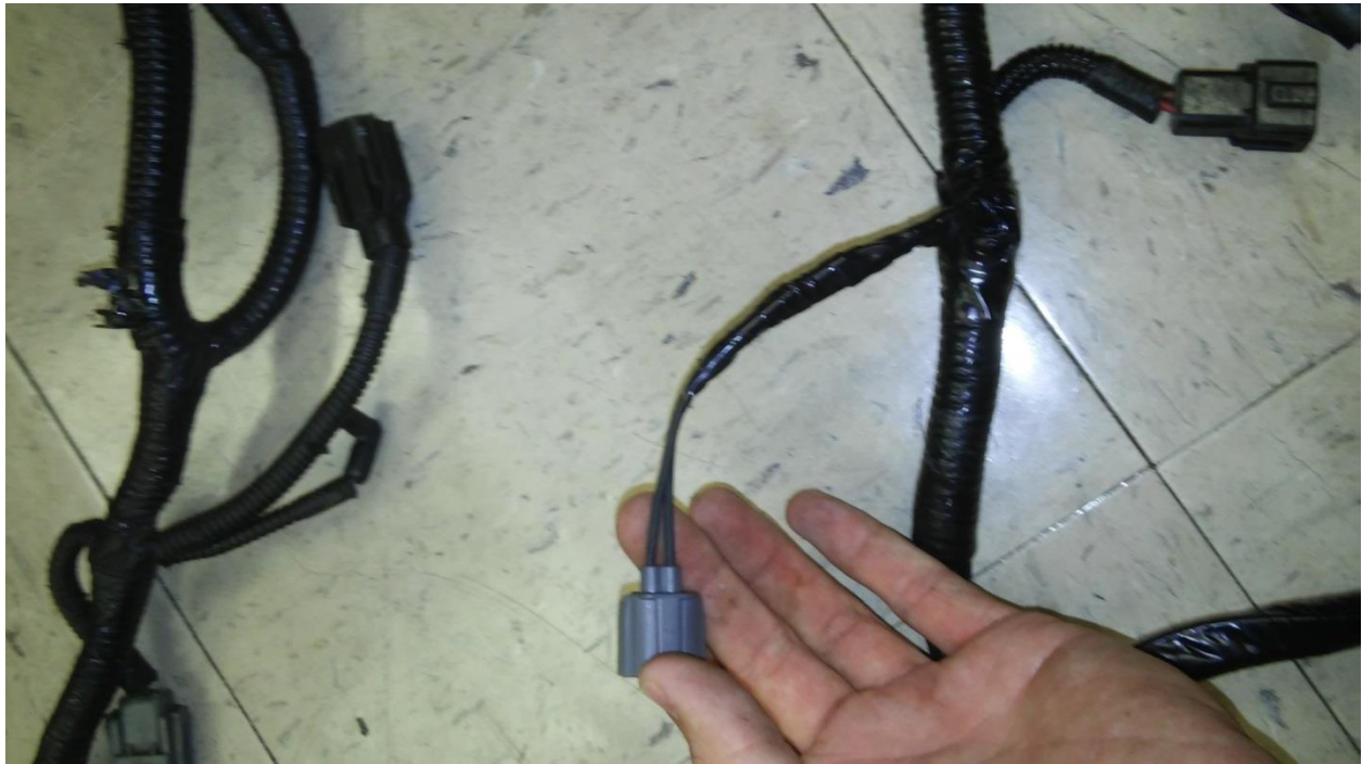
FIG A7.35 Aftermarket (TEI) coolant temp sensor connector pigtail installed.
