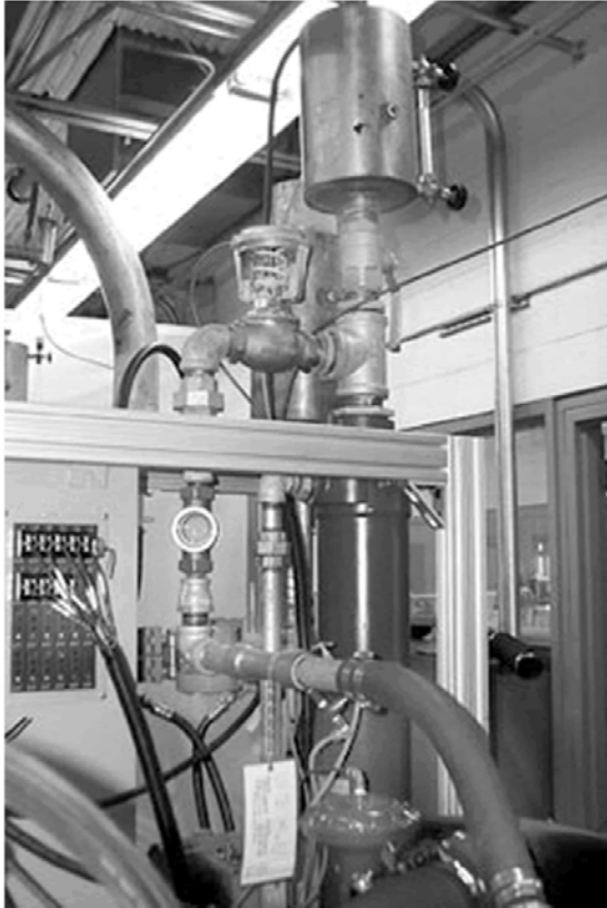
FIG. A7.23 Typical Cooling System, Flow Control Valve, Venturi Flowmeter, Reservoir and Sight Glass
