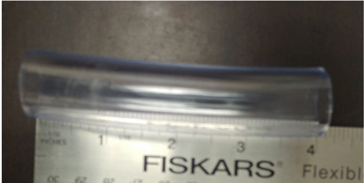
Oil separator side hoses, 2 each, 4 inches long.
