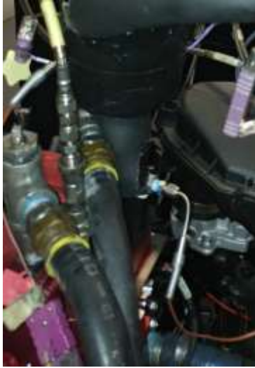
Fig. A8.26 Shows lower hoses wrapped with insulation.
