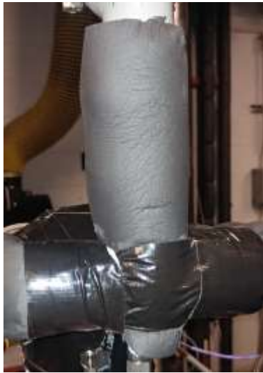
A8.21 Illustrates the wrapping of the upper part of the oil separator
