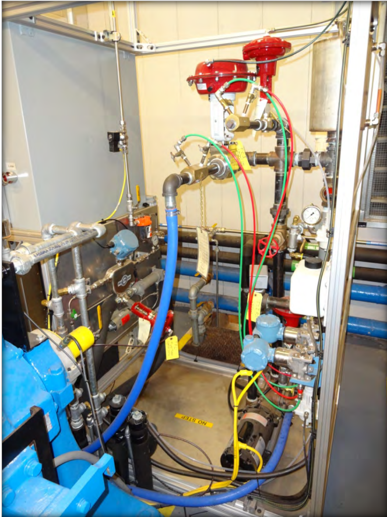
Fluid Conditioning Rack
