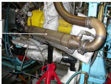
Heat Exchanger for controlling EGT
