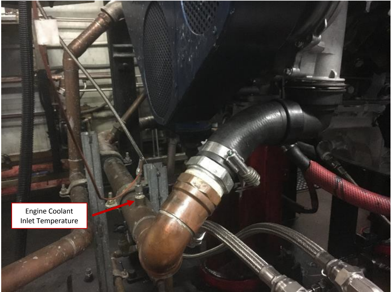
Figure A4-24 Engine Coolant Inlet Thermocouple Location
