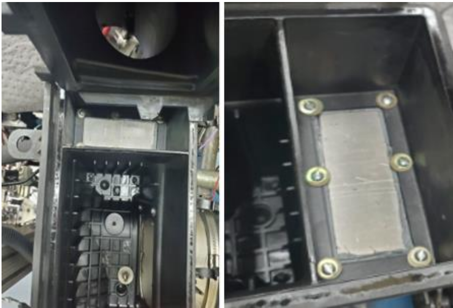
Figure A4.41 Alternate Air Inlet Blocked and Sealed
