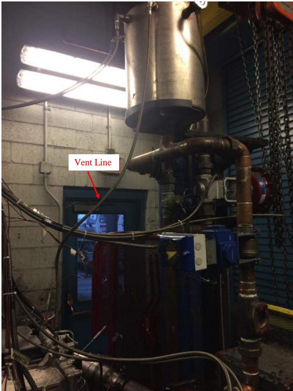
FIG. A4.2 EGR Cooler Vent Line and Coolant Tank
