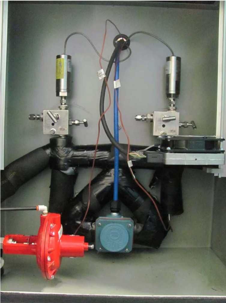
FIG A7.2 Aeration Measurement System and Enclosure
