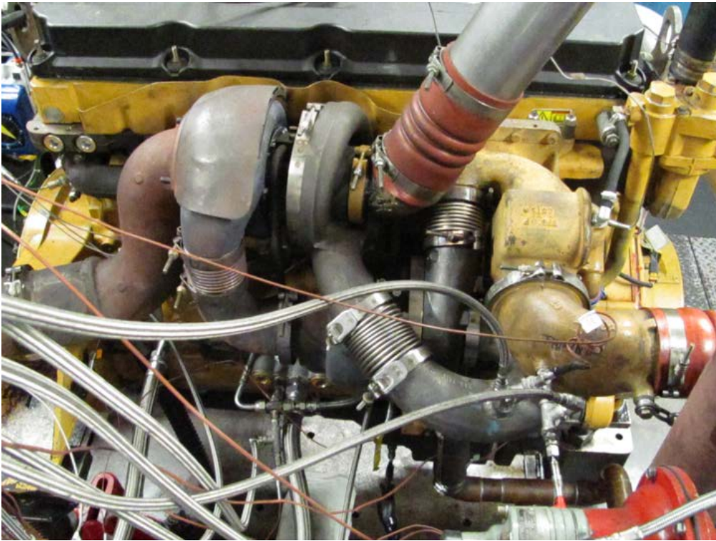
FIG. A5.19 Right-Hand Side of Installed Engine
